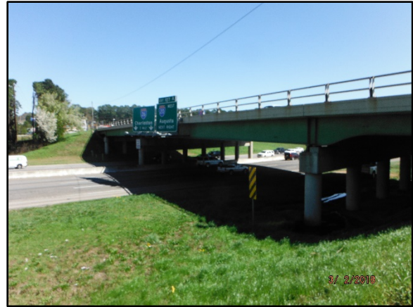
Photo 1 – View of the subject bridge, S-32-36 (St. Andrews Rd.) Bridge over I-26 looking up-station (Westward).
